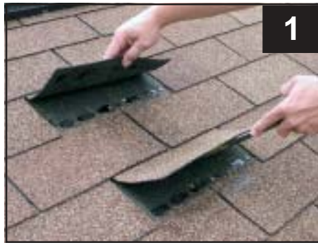
1 Locate truss with stud finder, lift shingles with prybar at dish location, do not lift middle row
